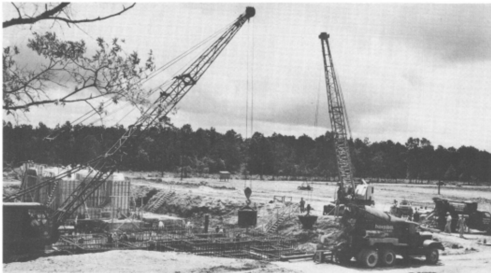
This 1948 photo shows the pouring of the concrete for the Greens Bayou No. 2 turbine-generator foundation.
