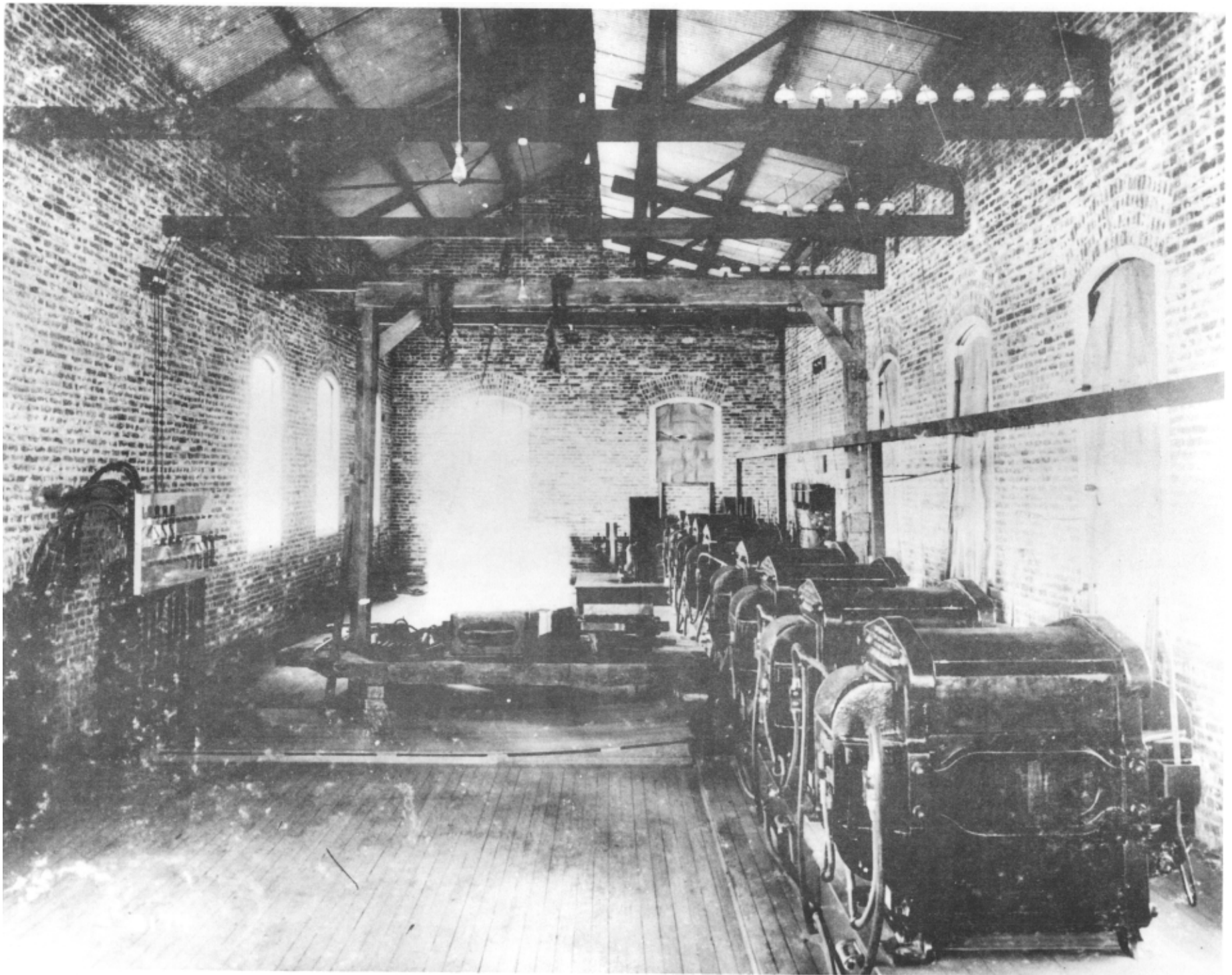
A view of the original 12 air-blast transformers, later replaced by Westinghouse transformers.
